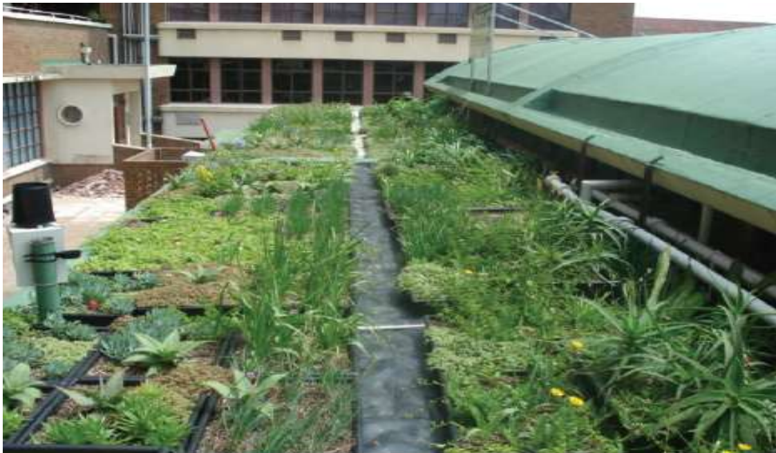
Figure 2.2: eThekweni Green Roof Pilot Project, Durban CBD ((Greenstone, 2010).
