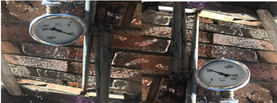
Exhibit 7: Pressure tower near reservoir
