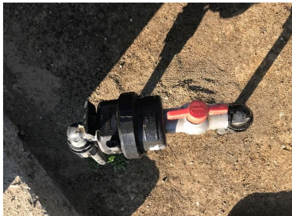
New replaced water meter
